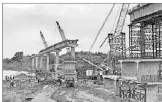
The site of the Hamirpur bridge collapse on Friday.
